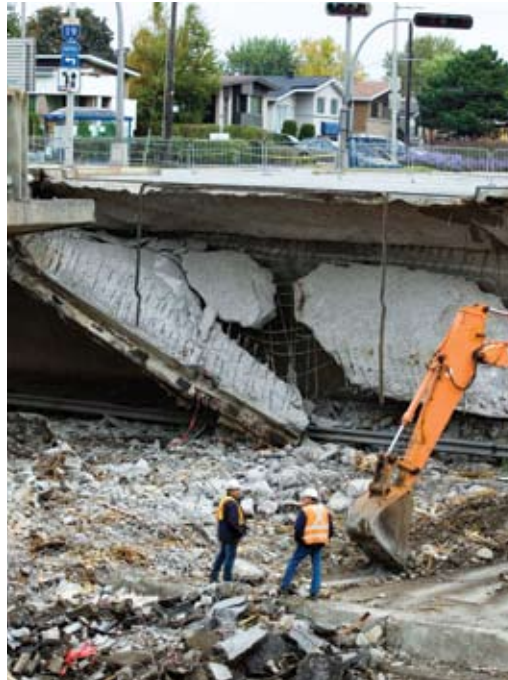
Rebuilding an overpass that collapsed in Laval, Quebec, in 2006 took money as well as muscle. Canada’s cities face shortages of funds for replacing major parts of their aging infrastructure.
